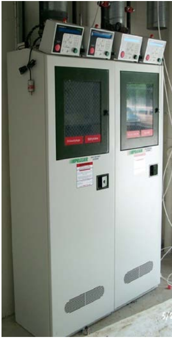
Figure 2: Automated-purge gas cabinets used in BNC. These cabinets are required for all gases rated 3 or above in any NFPA hazard category. The cabinets are located in secure, isolated rooms at the perimeter of the facility. In addition, each cabinet is locked to provide further security.
