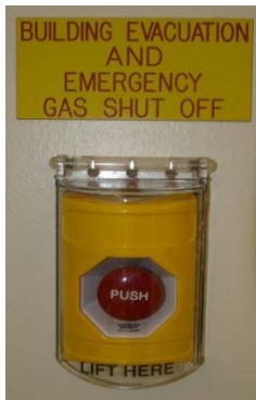
Figure 4: In the event of an emergency being recognized by a facility occupant, push-button stations allow one-touch evacuation of the facility and gas shut-off.
