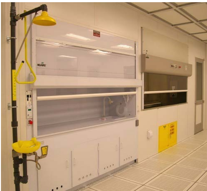
Figure 1: Acid and solvent fume hoods bulkhead-mounted in the BNC cleanroom. Bulkhead mounting equipment allows the separation of the operational side of the equipment (shown) from the maintenance side of the equipment, accessible through the cleanroom chase.
